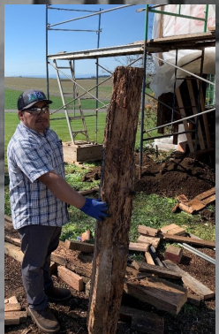
Ioka employee Efrain Hernandez holding a rotten sill board.
