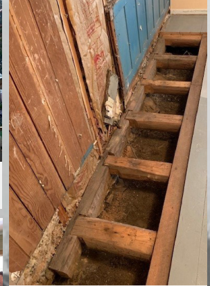
Floor joists in old original bedroom. All logs are hand hewn, notched, and set with no nails.
